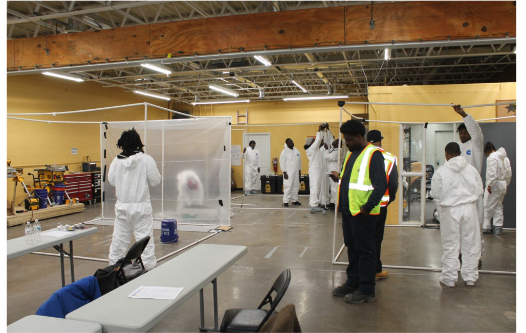
Flip the Script participants working in small groups to build a asbestos containment.
